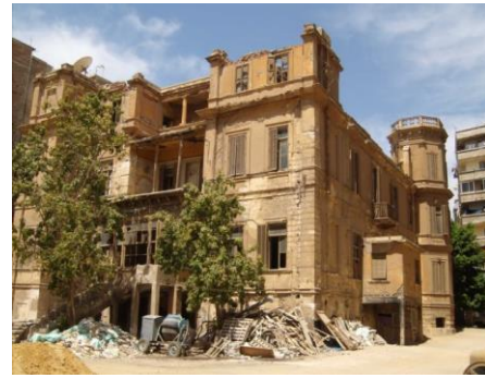
Figure 2. The villa of the architect Aldo Ambron that was used as house of the great British author Lawrence Durrell demolished.
